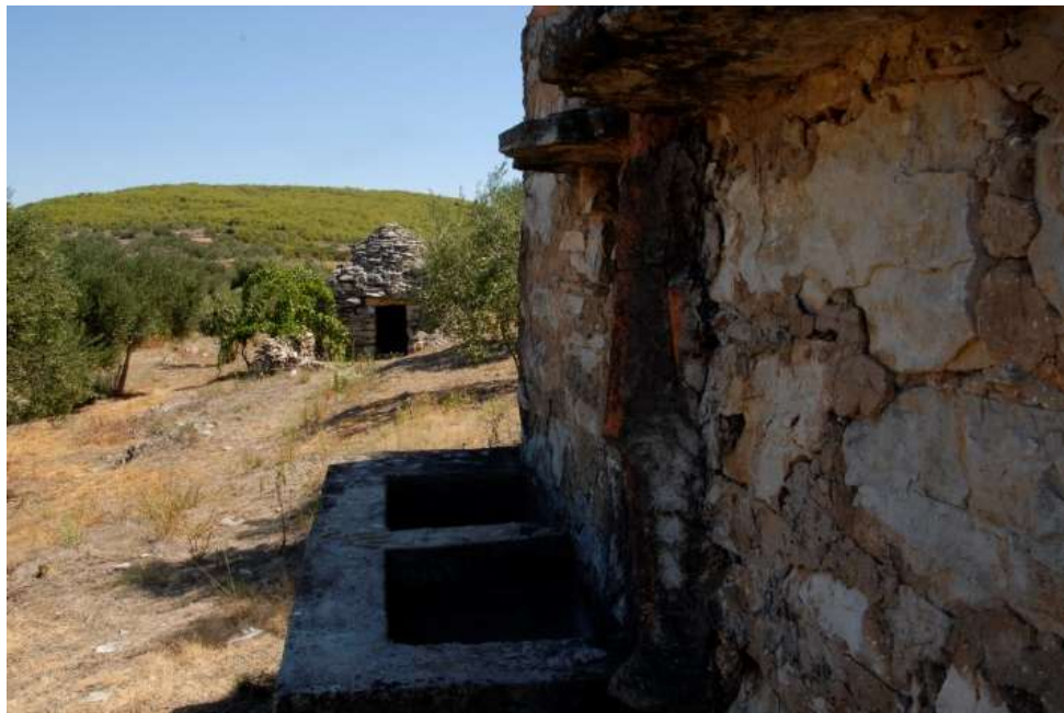
p 4.10: Longitudinal toreta is an interesting object in stone, high and equipped with yards and stone details: water bowls, lintels, openings. There are still five toretas on the high plain of Korčula island.
