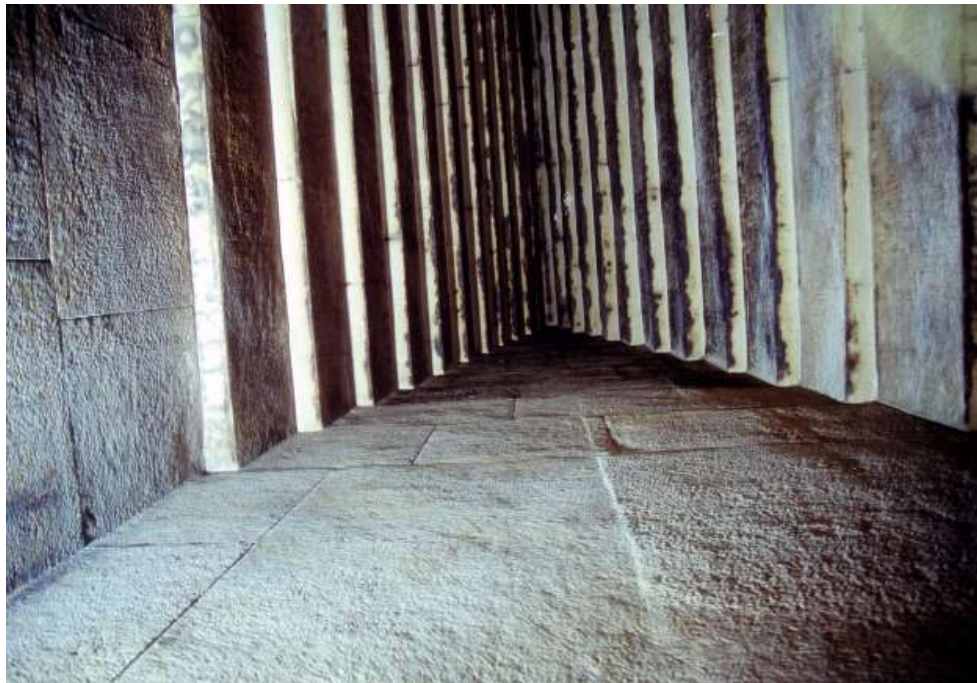
p 1.1: Corbelled construction can be found in Bent pyramid – longitudinal corbelling appears in burial cells, second Millennium BC.
