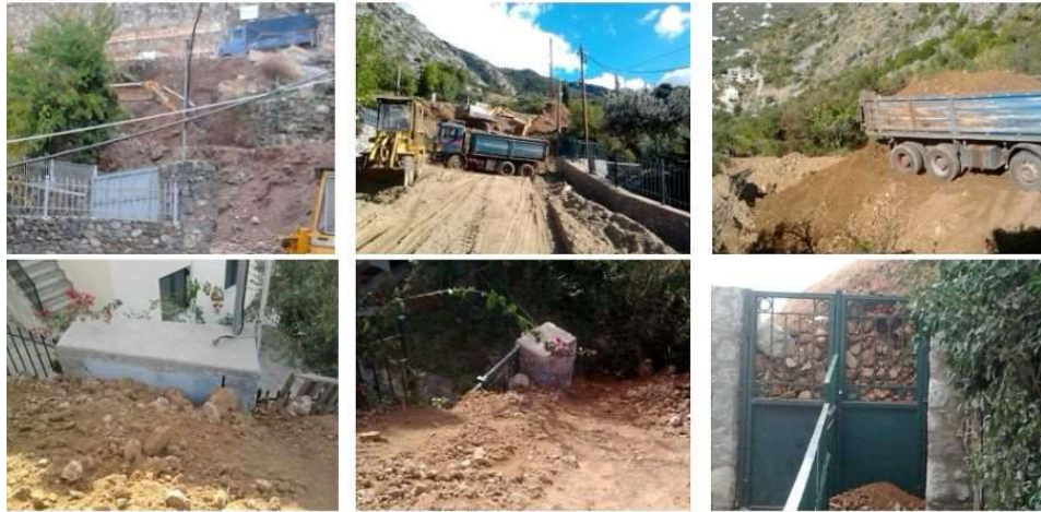
CONTRACTOR’S ARBITRARY AND ILLEGAL ACTIONS
