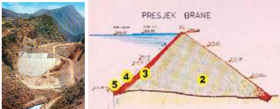
Figures 12.-13. Rock filled concrete faced dam “Rama” under construction (left); Cross section of the dam with dry-stone wall (“3”), located between the upstream reinforced concrete facing (“4”) and the rock embankment of 1,4 million m 3 volume (“2”)... (right) 18
