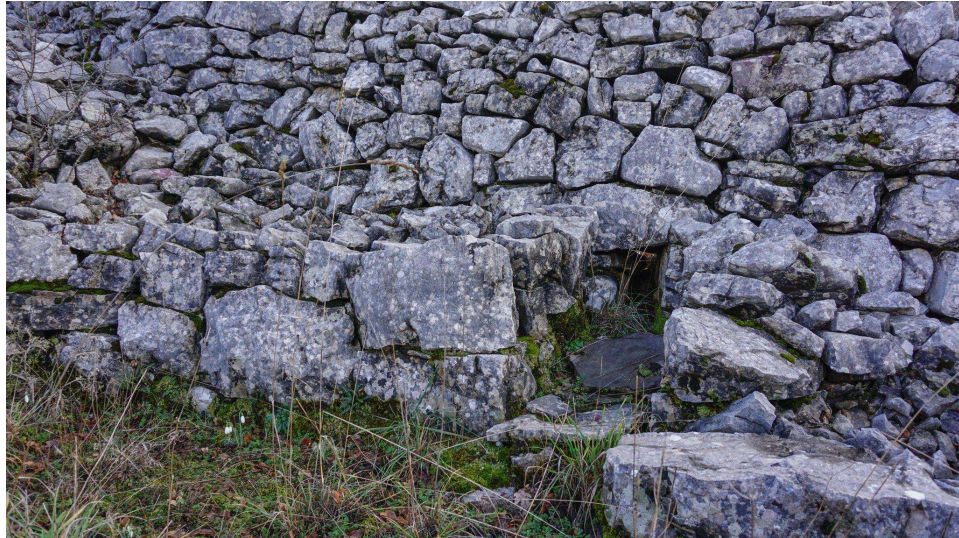
Figure 12: Conduit in Duba Konavoska
